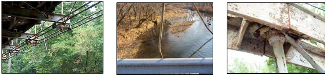
Figure 8: (a) Lower chord loops are generally in good condition, but note the broken diagonal rod; (b) Bent vertical and diagonal rods; (c) Example of a severed diagonal rod.
