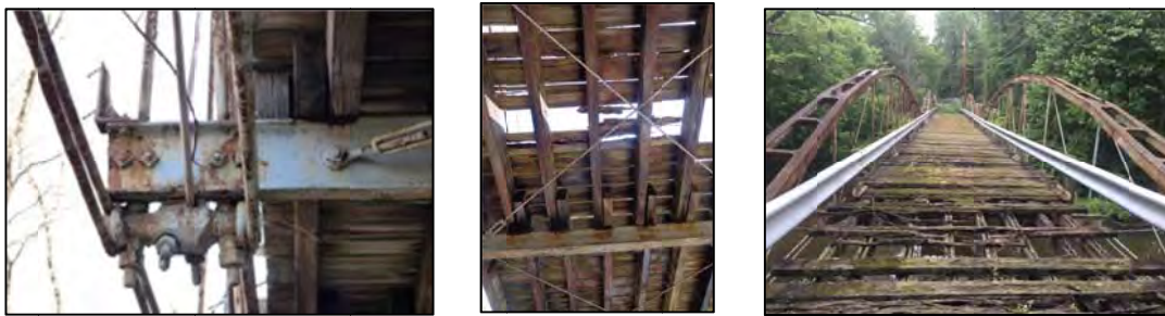
Figure 9: (a) Detail of beams and junction blocks typically in good condition; (b) Detail of diagonal floor bracings and deck from below; (c) Condition of deck from above.
